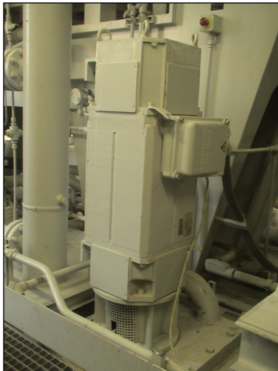
Emergency oil pump
