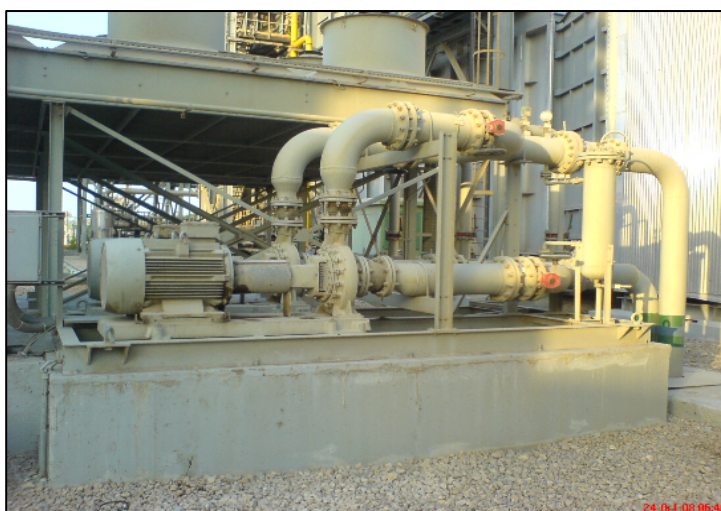
Cooling water pump motor
