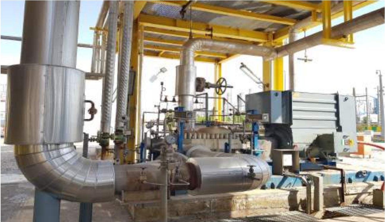
Feed Water Pump & Fcv-01-F
